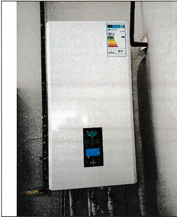
Pic.1 - General view of the E300 boiler.
